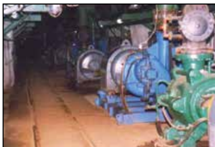
Bank of dewatering pumps.
