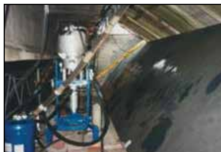
Pitting repaired using ARC 858.
