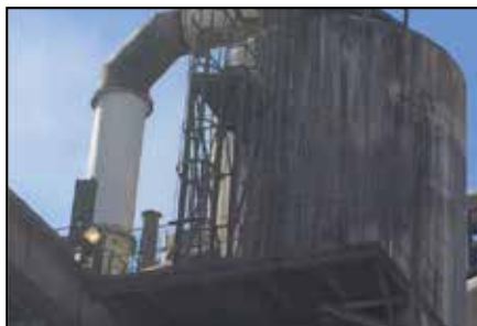
Flash cooler with exhausters.
