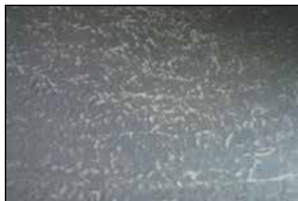
Corroded tank internal surface.
