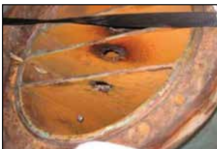
Corroded divider plates.
