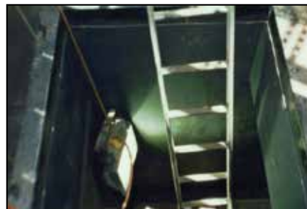
ARC specified by plant engineer.
