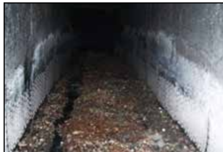
Discharge flume with damaged tile/rubber liners.
