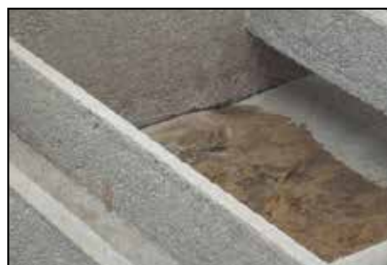
Drained sand filter vessel.
