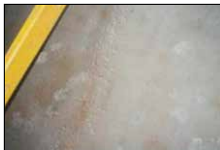
Corrosion and pitting on the spillway gate.
