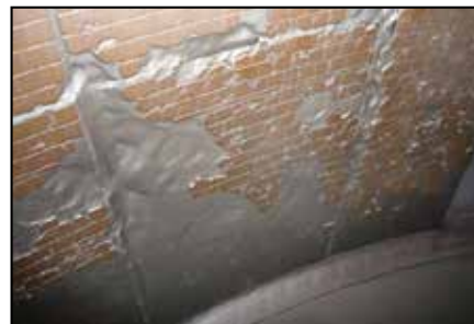
Damaged pulverizer walls.
