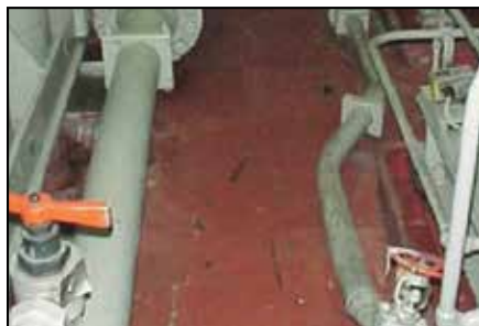
Previous coating one year after installed.
