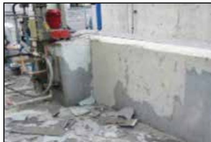
Failed coating after spills.
