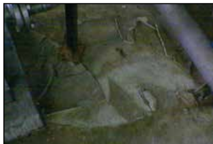
Delaminated fiberglass mat polyester.
