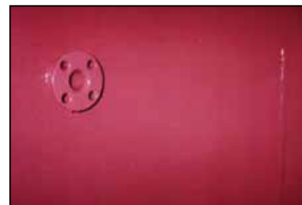
After proper surface preparation, ARC S4+ was applied in a two-coat system.
